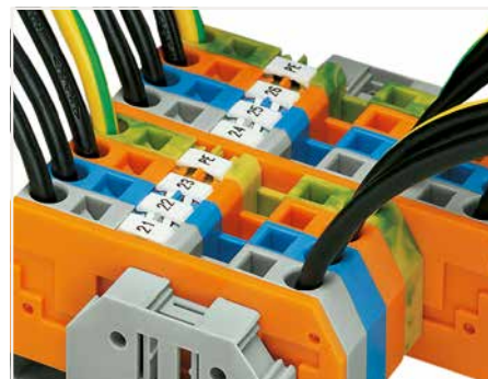
The markers are not covered by the wiring when marking terminal blocks in center position.
